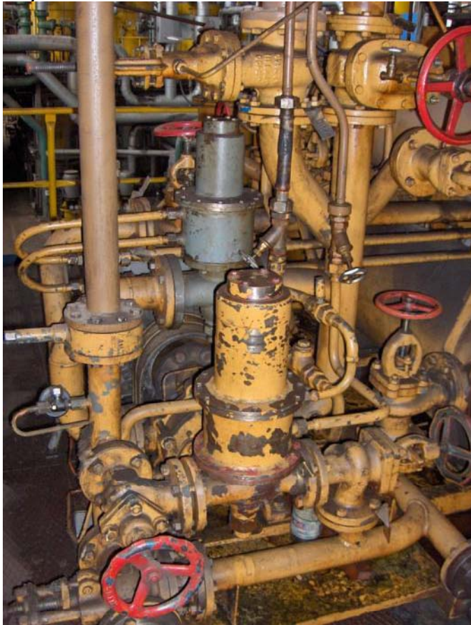
Oil system before
